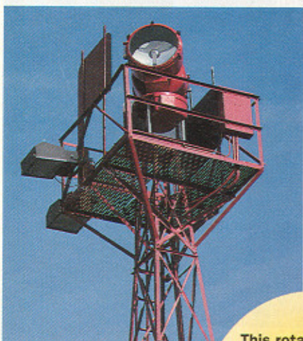
This rotating beacon, currently in service at the Santa Monica (California) Municipal Airport, is actually in its second career. The beacon and its tower first served on an airway.
